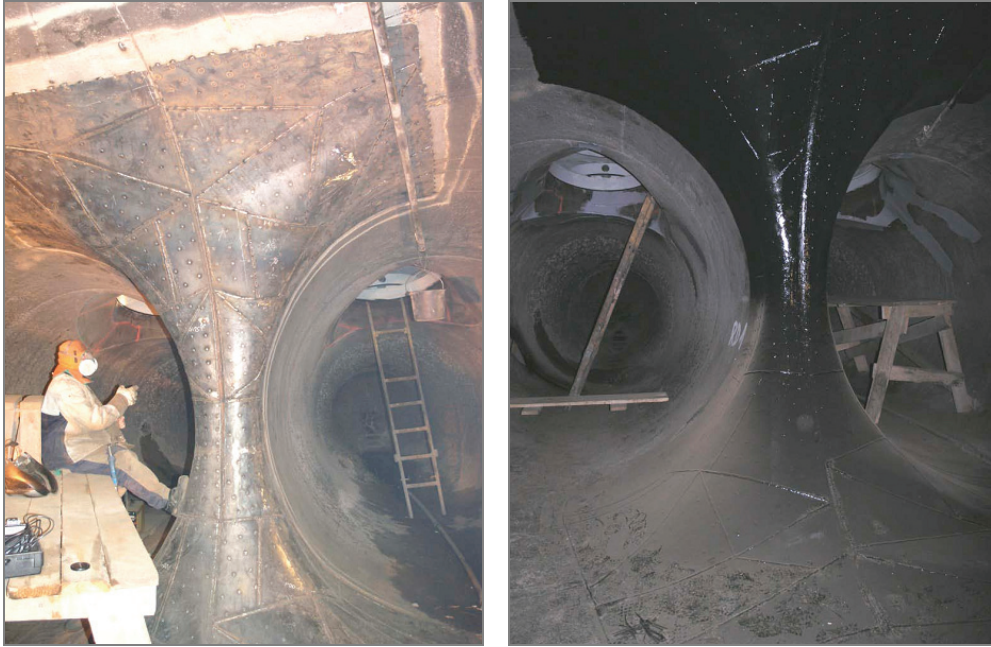
Fig. 17. Structure welding of the reinforcement components to the coating of the pipeline branch and the completed painted plating of the pipeline branch.
