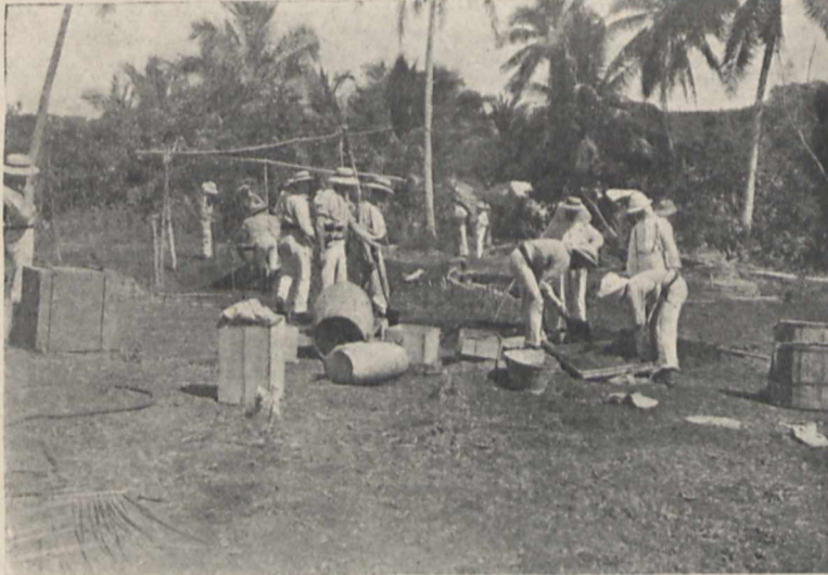
FIG. 3.—Preparing concrete for the pillars. Sand, cement, and dead coral (the last-mentioned quarried from the top of the hill) were used.
