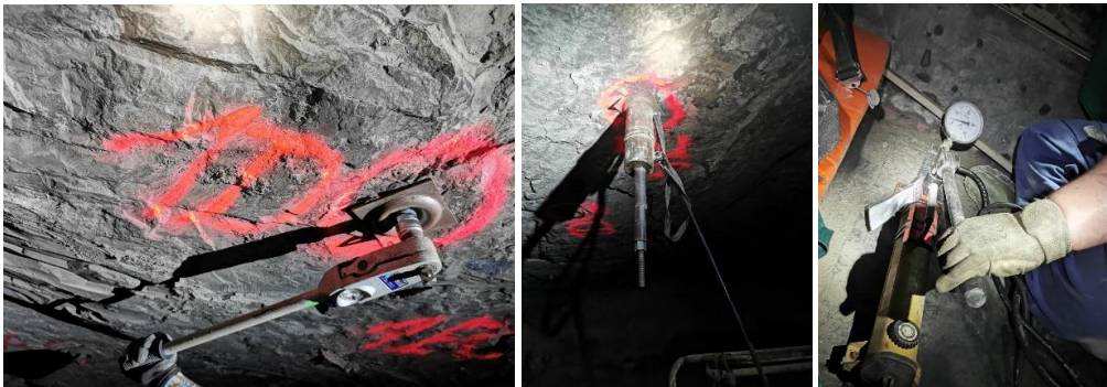
Fig. 5. From the left: 1) checking the bolt tightening torque with a torque wrench, 2) cylinder with sleeve, 3) hydraulic dynamometer pump (own photos)
