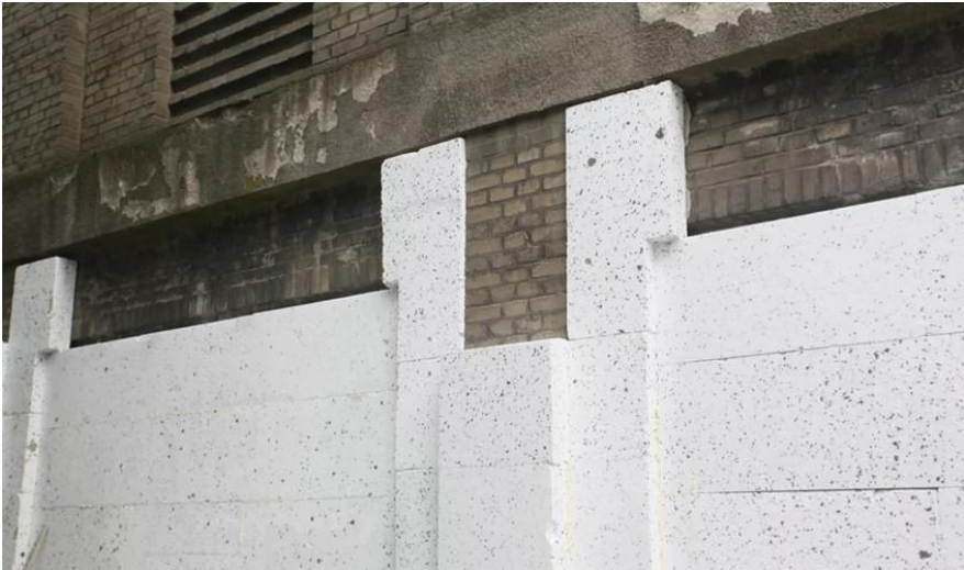
Fig. 5. View of the facade of the K. Szpotkański factory during thermo-modernization works in 2015.
