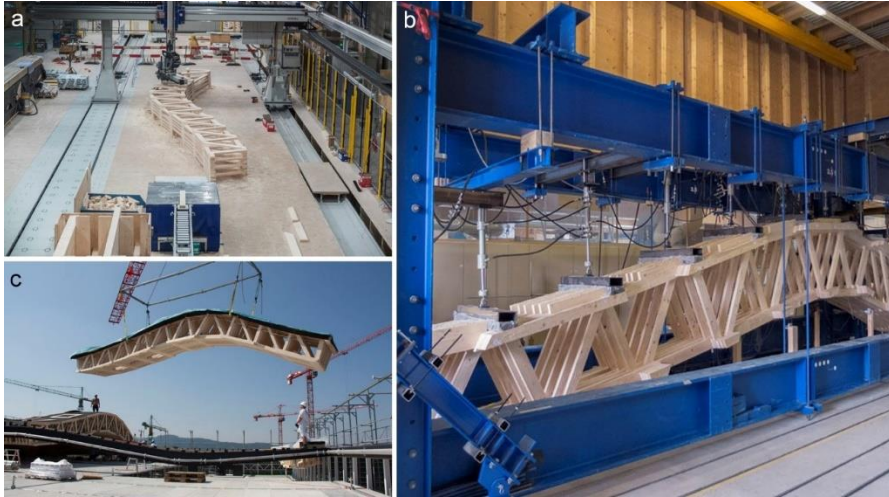
Fig. 5. The Sequential Roof of the Institute of Technology in Architecture, ETH Zurich, design by Arch-Tec-Lab AG and manufactured by ERNE AG Holzbau, 2016: a, b – structural element in automated production, c – ready-made prefabricated element during the assembly of the structure; source: a)–c) photo by Gramazio Kohler, “ETH Zurich – ITA Institute of Technology in Architecture”, Arch_Tec_Lab/ Roof, < https://ita.arch.ethz.ch/archteclab/sequential-roof-.html/ > [accessed: 20.05.2021]
