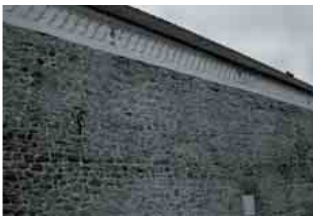
Fig. 9. The west part of the cloister walls from bishop Radziwiłł's time with junction of walls, the so-called toothing, after the preservation in 2008 (photo: O.M. Przybyłowicz)
