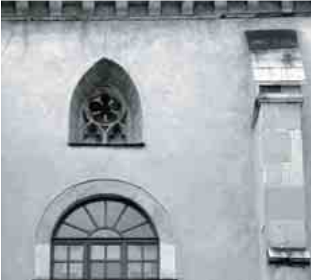
Fig. 6. Outer arrangement of the north elevation of the monastic church, with a 2. half of 13 th . c./1. half of 14 th c. traciery and the new window of the 17 th c. (photo: O.M. Przybyłowicz)
